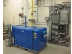
THE CHP SYSTEM AT NORTH HILL PROVIDES ELECTRICITY, SPACE HEAT AND DOMESTIC HOT WATER.
