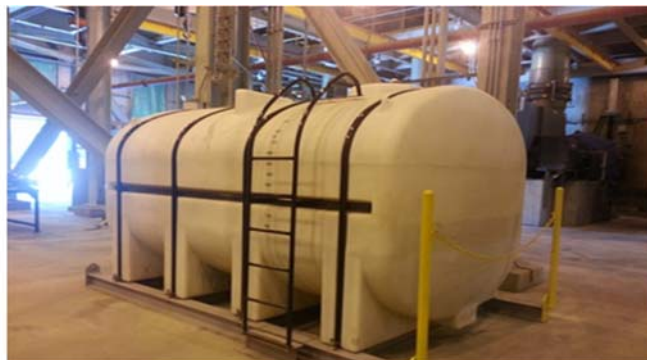
SA2 is available in tank truck quantities for bulk storage (as shown above) and in 265-gal totes.
