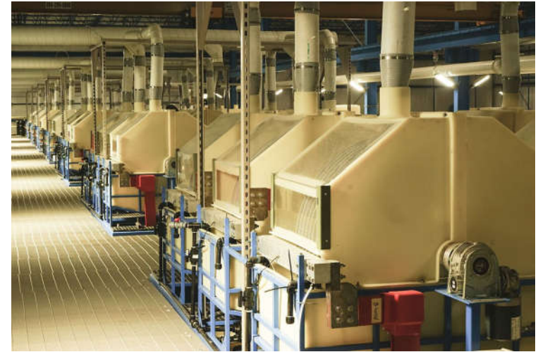
Aqua Metals' AquaRefining Modules at its TRIC facility
