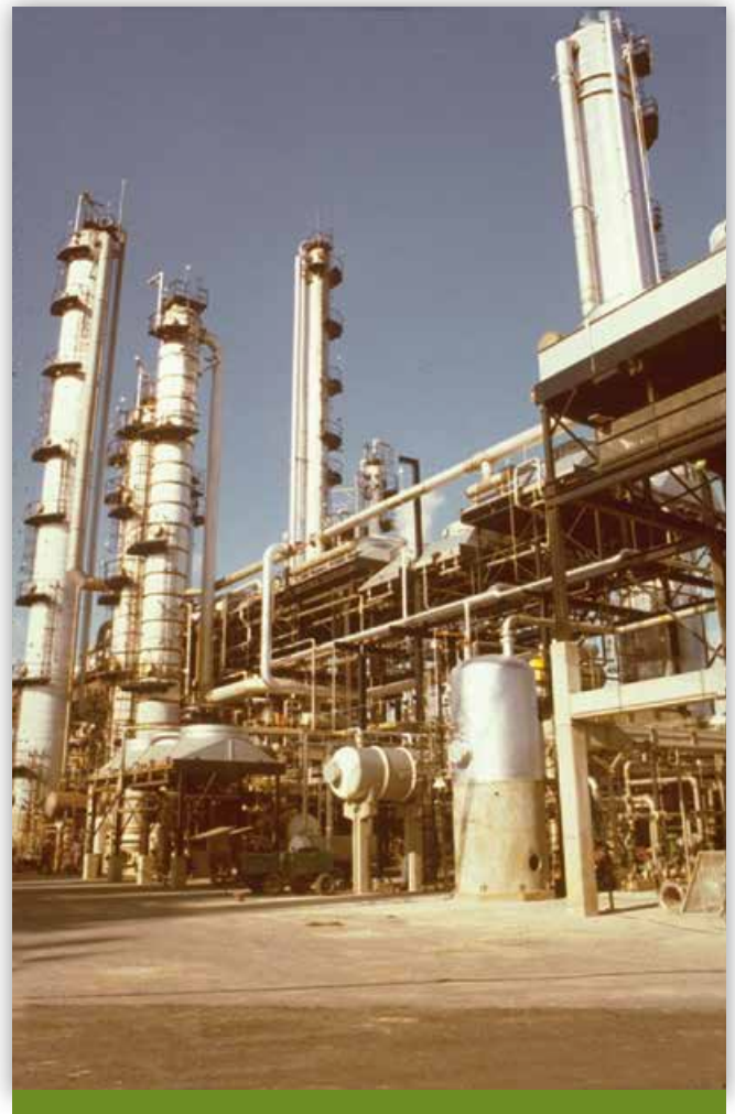
Concern for hydrogen-induced cracking (HIC) susceptibility of plate steels used to fabricate vessels for processing petroleum and petrochemicals significantly increased the demand for the low-sulfur levels with shape control offered by FINELINE® steels.
