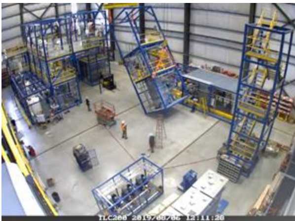
Phase 1 & 2 Modules Being Disassembled and Prepared for Trucking – clip from video taken Aug 06th, 2019
