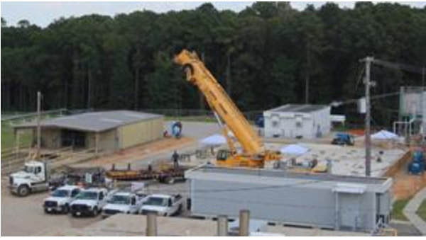
Project Site Location Showing Completed Foundations and Mobile Crane Ready to Install Modules – Image taken Aug 21st, 2019
