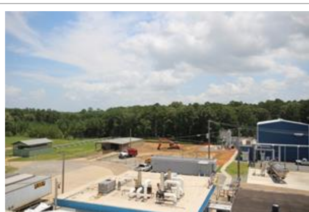
Standard Lithium; construction begins at El Dorado, AR lithium extraction demo plant
