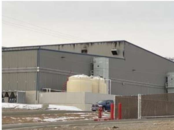
Flames inside the AquaRefining area reached the roofline.
