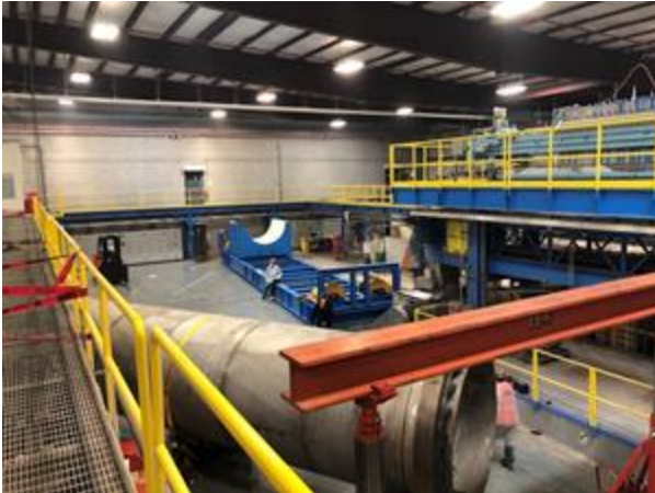
Figure 1 – Part of Phase 2, the drying system arrived and was recently rigged into place in August (during a safety stop) adjacent to the Phase 1 filter press and is now undergoing installation and commissioning
