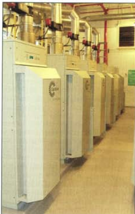
Figure 1: Twelve Capstone C65 Hybrid UPS microturbines are installed in Syracuse University's Green Data Center. The center is designed to use 50% less energy than traditional data centers
