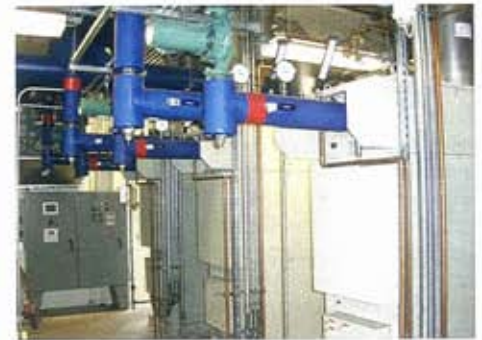
Janesville installed four 65 kW Capstone microturbines (top) equipped with integral heat recovery. The circulating hot water supply and return connections on the heat recovery module are shown above.
