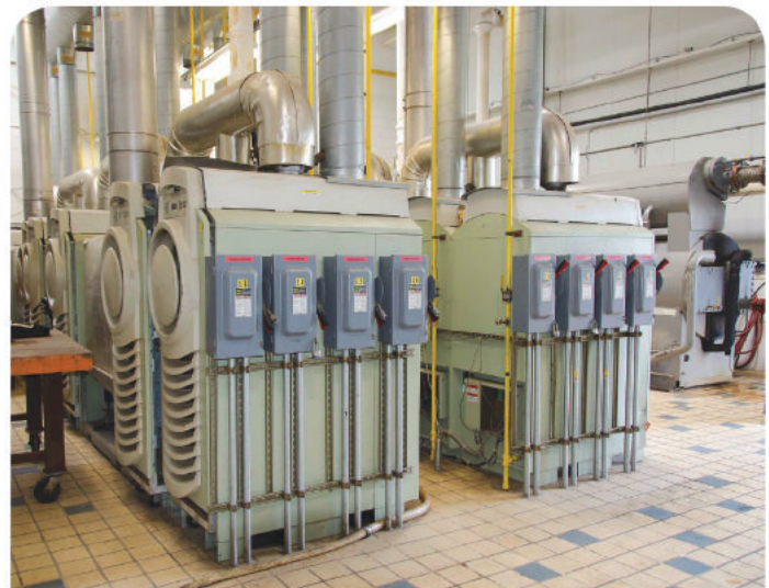
These natural-gas micro-turbines generate both electrical power and hot water for heating and cooling the plant. Bechtold calls it Combined Heat and Power (CHP).
