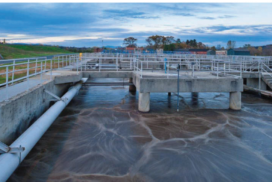
Aeration basins at the Pittsfield treatment facility now use 150 kW turbo blowers (HSI Blowers) and fine-bubble aeration (Sanitaire).
