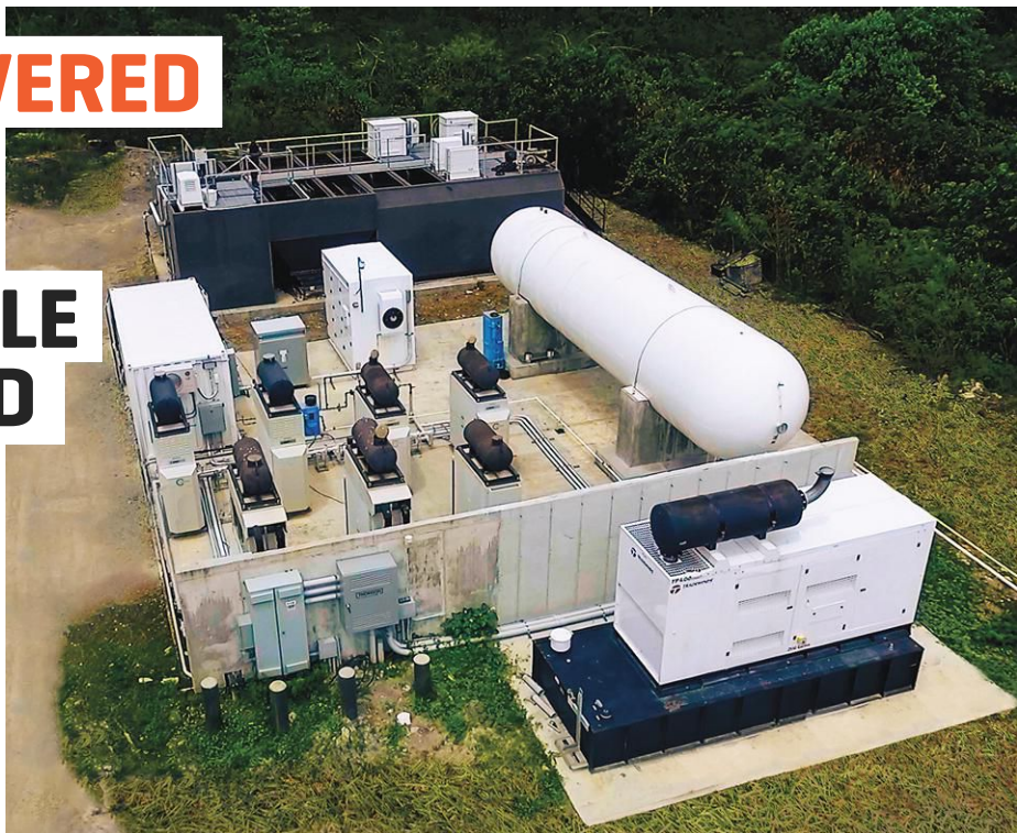
The Magens Junction microgrid is powered by seven propane-fueled microturbines. The 18,000-gallon on-site propane storage tank provides eight to 10 weeks of fuel autonomy before a refill becomes necessary. [Images courtesy of Capstone Green Energy.]
