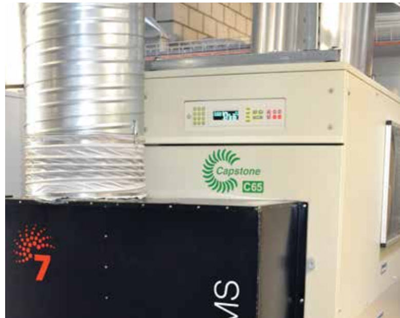
Twelve CR65 Capstone microturbines installed in a CHP application at the Gefu Produktions AG manufacturing facility in Lucerne, Switzerland, use milk sugar from the manufacturing process to generate onsite electricity and heat.
