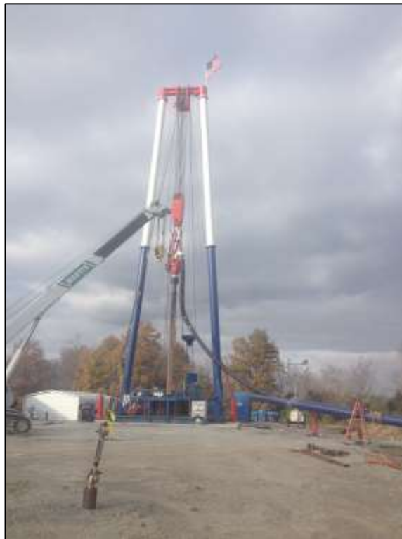
Example of Blind Drilling of Vertical Airshafts Similar to Poplar Grove Mine
