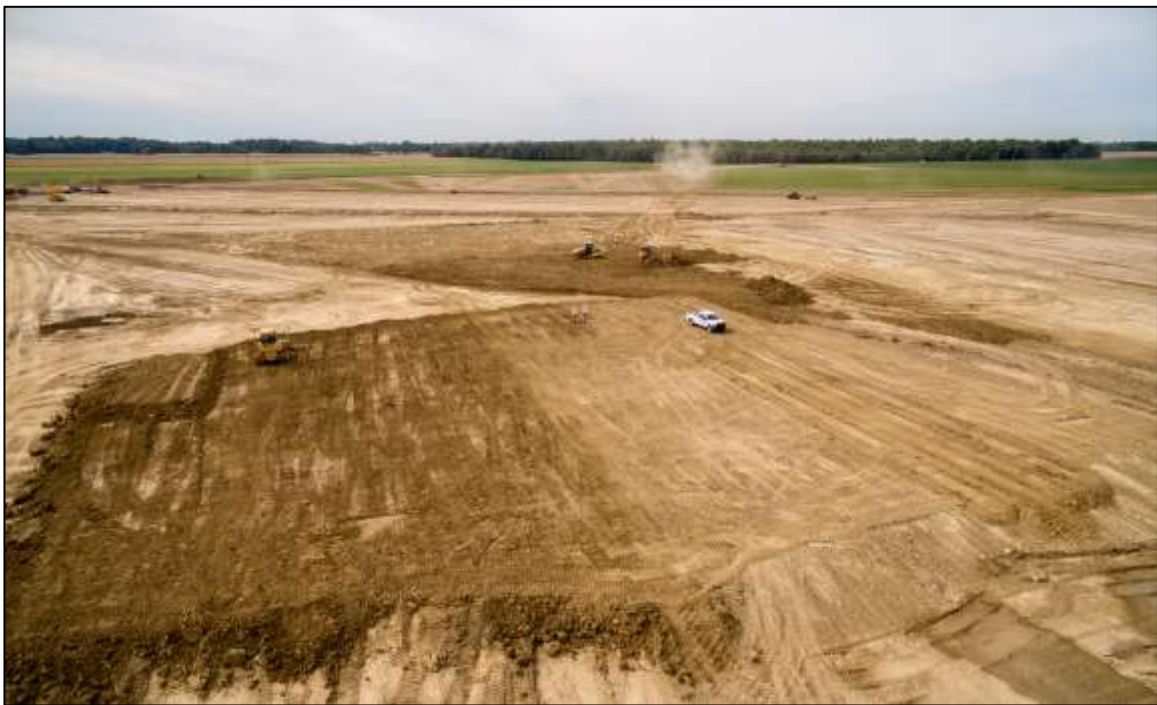
Site Pad Prepared for the Coal Handling and Preparation Plant ("CHPP") at Poplar Grove
