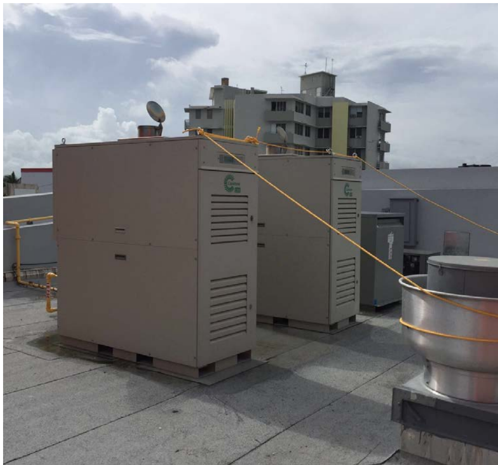
Capstone C65 Microturbines on the Rooftop of a Popeye's Restaurant in Puerto Rico
