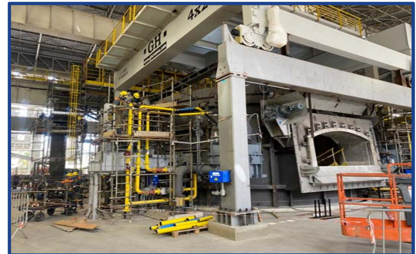
Guthrie pre-treatment and Pinda recycling melter lines
