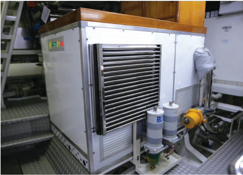
INSTALLED ON BOARD LETHANTIA
