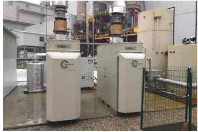
Two Capstone C65 microturbines ensure high reliability while also benefiting the environment.
