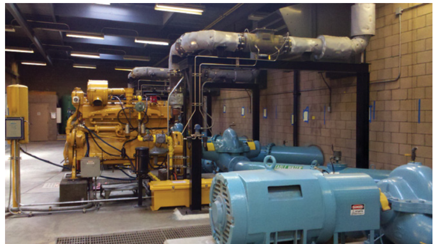
The Ultra Emissions System is designed for installation on rich-burn natural gas engines to meet stringent emissions standards, Tecogen said. This system was part of a pilot project at the Eastern Municipal Water District in Perris, Calif. It was installed on a 15 L Caterpillar natural gas engine used to move stored water.
