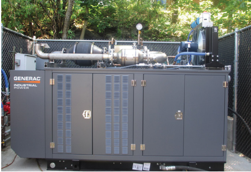
Tecogen's Ultra Emissions System, shown here during testing, is a patented turnkey retrofit kit that the Massachusetts-based company has begun to market.
