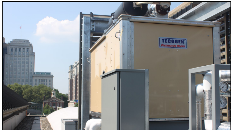
The Tecogen CM-75 cogen module on the roof of the Independence Visitor Center with Philadelphia's Independence Hall in the background.
