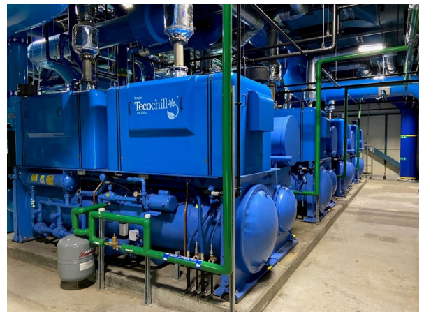
Tecochill plant located on the University of Connecticut's main campus central plant. Four DTx-400's provide 1600 tons of cooling.
