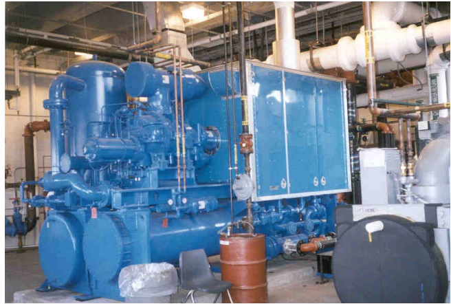
A Tecochill CH-500 unit installed on site at South Campus since 1998 and has been maintained by Tecogen's factory service center in East Windsor, CT for the past 25 years.
