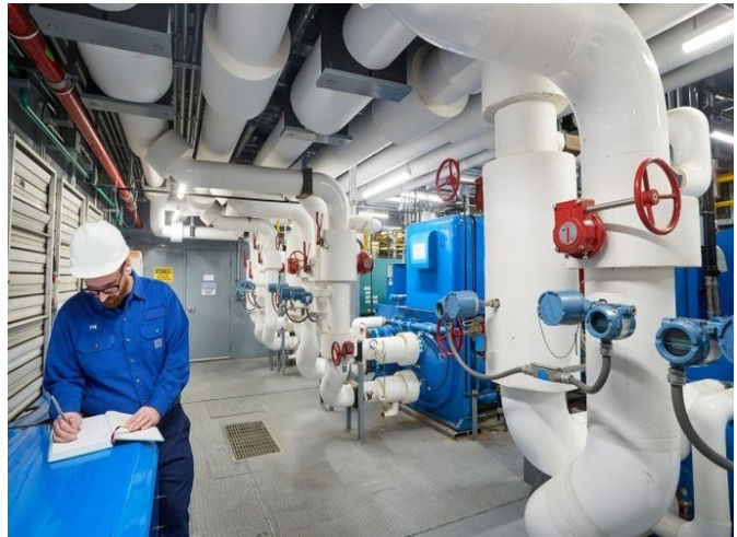
The Tecochill units fully installed on site at TWA Hotel in Queens, NY.
