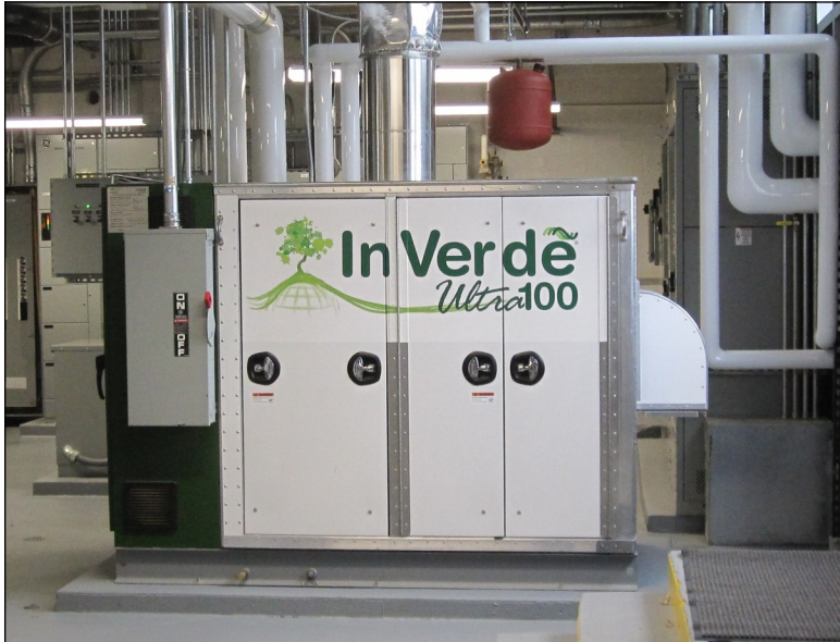
Seaford High School's addition and renovation project at received the Energy Solutions Center's 2013 Partnership Award for Innovative Energy Solutions. Tecogen's InVerde Ultra 100 cogen module is a key feature of the project.
