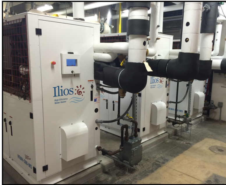
Seven (7) Ilios HEWH-500-WS units provide simultaneous heating and cooling to keep the Institute at the proper climatic conditions for their research needs.
