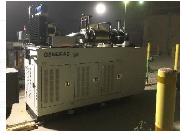
Natural Gas Generator Upfitted with Ultra in Southern California (LA County)
