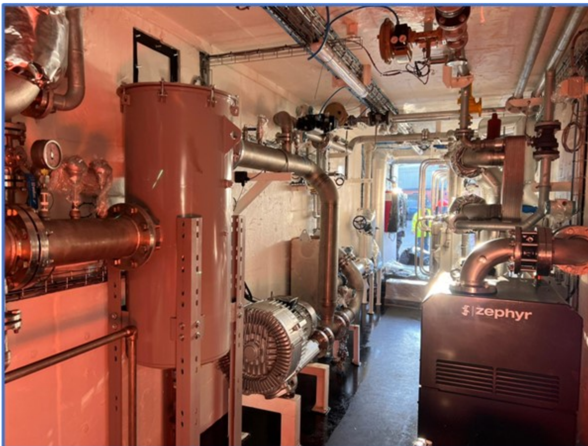
Figure 1: Inside the Carbon Capture Pilot Plant during commissioning prior to shipping. Following construction by Aqualung, the plant was shipped from Wales, UK to Galveston, Texas, and then transported to the plant location in southern Arkansas.
