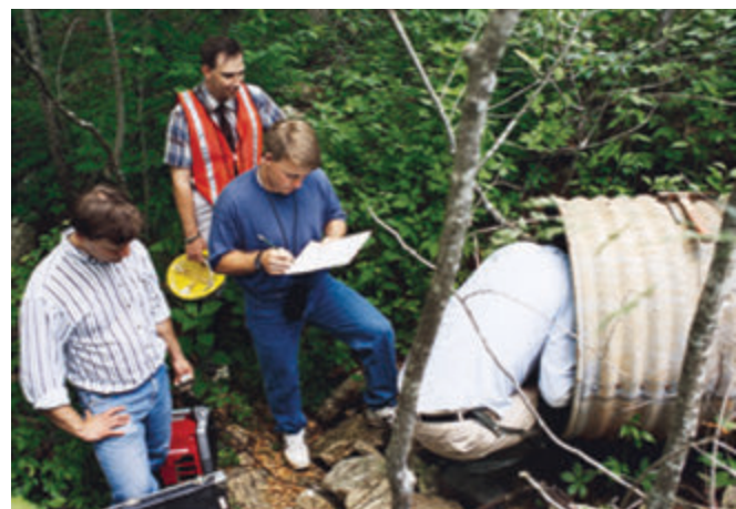
Cleveland-Cliffs Research Center's corrosion engineers and Missouri DOT material engineers inspect a 43 year old Aluminized Steel Type 2 pipe installation. This is one of two culvert installations in Carter County, Missouri, installed in a series containing half Aluminized Steel Type 2 pipe and half galvanized steel pipe.
