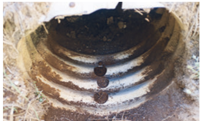
This Aluminized Steel Type 2 corrugated steel pipe was installed in 1953 in El Dorado, California. It was inspected in 1982, 1995 and in 2005. Coupons were removed for evaluation by the Cleveland-Cliffs Research Center and CALTRANS.
