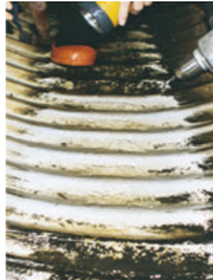
This close-up view shows the Aluminized Steel Type 2 pipe installed in Garland, Maine, with the dark staining wiped away to reveal the like-new underlying aluminum
