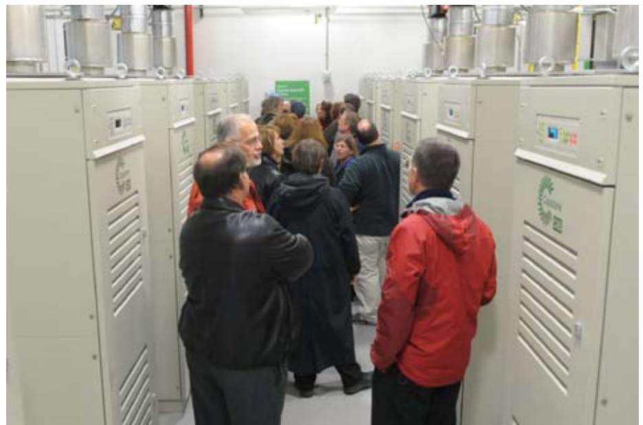
There are 12 Capstone microturbines providing energy for the Syracuse data center.
