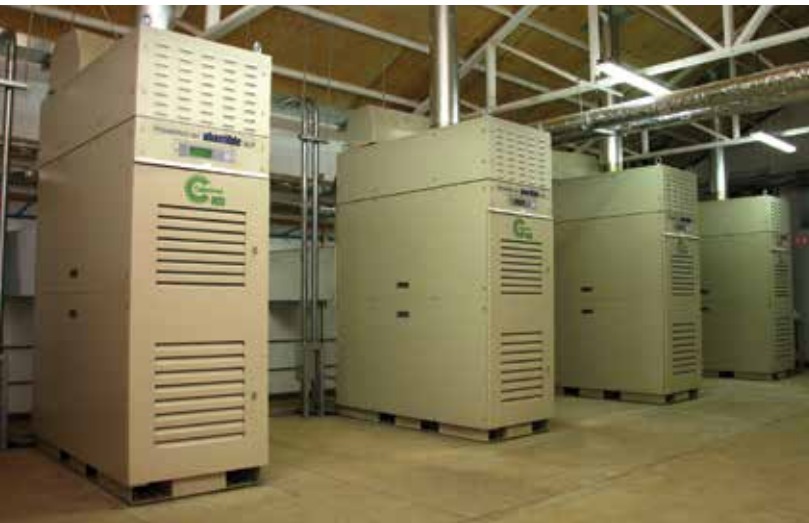
The cogeneration system supports 100 percent of power demand for this luxury hotel and is capable of delivering 1,752GWh of electricity and 3,504GWh of thermal energy per year at full load.
