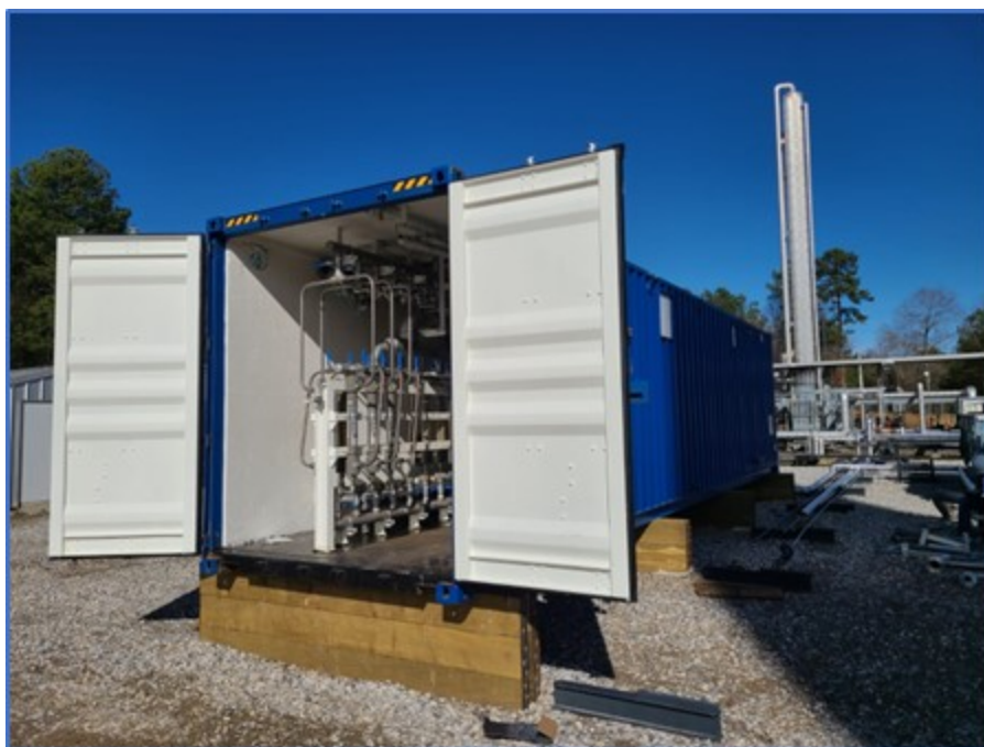
Figure 2: Initial installation of the Carbon Capture Pilot Plant at the testing site in southern Arkansas. The plant is located at a natural gas processing facility and will be used to assess the feasibility of CO 2 capture from natural gas burning flue emissions.
