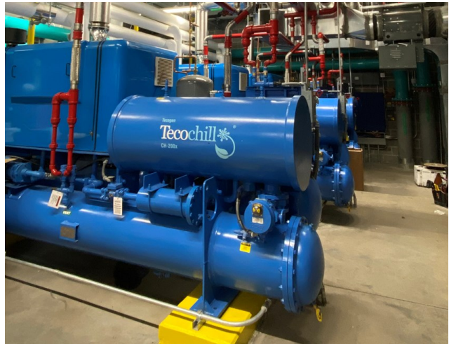
Tecochill plant located at the Skating Club of Boston. Five CH-200x chillers make up to 1000 nominal tons of cooling to produce ice for three rinks and air conditioning.
