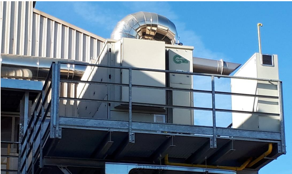
Capstone C200 microturbine installation. Source: www.capstoneturbine.com
