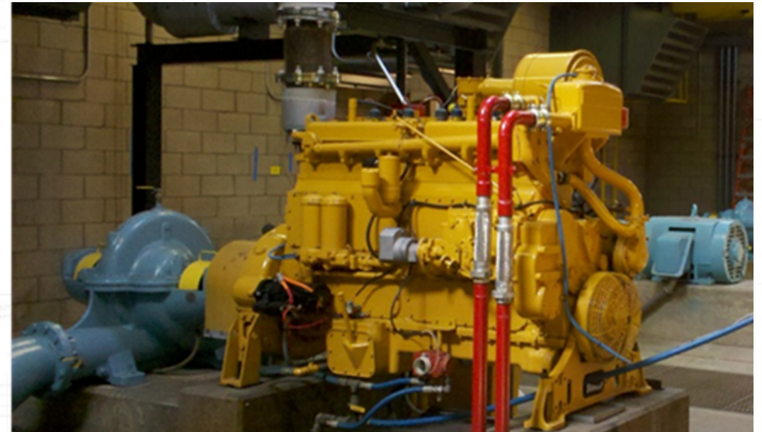
Ultra equipped 300 HP water pumping natural gas engine
