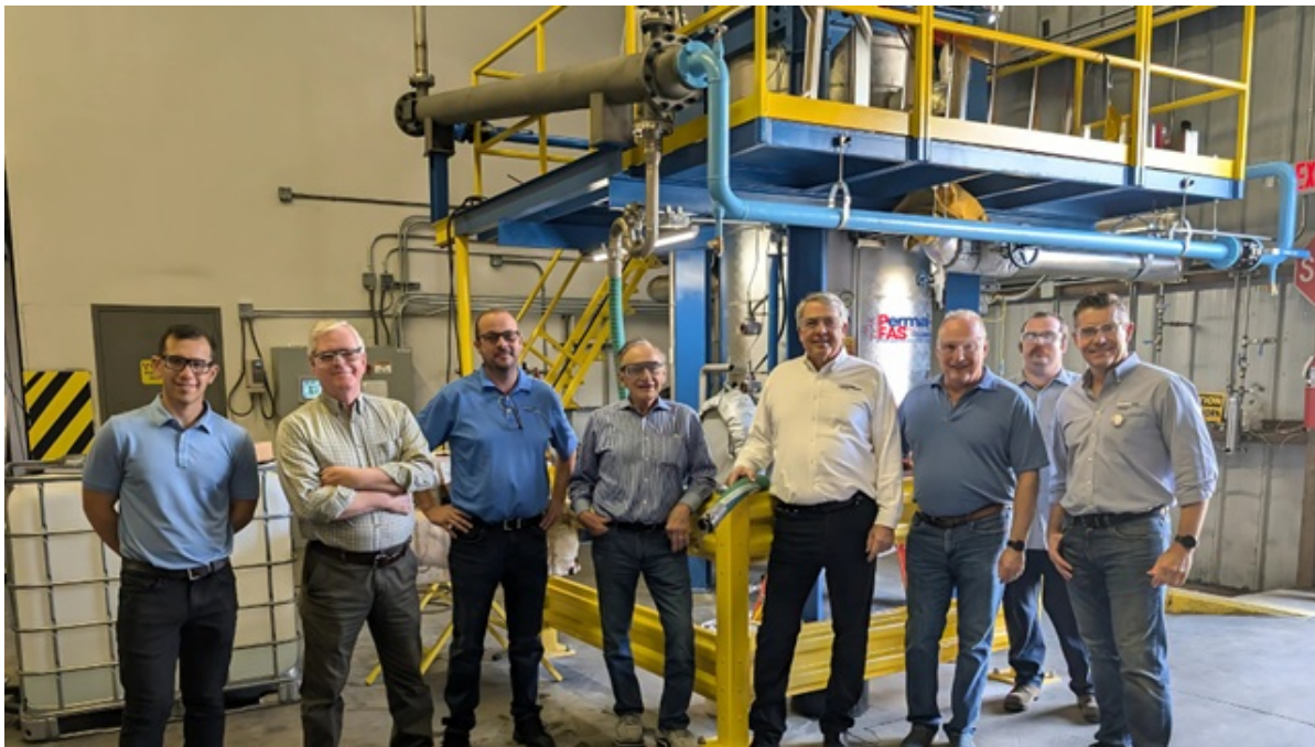
First Commercial Perma-FAS System for PFAS Destruction
