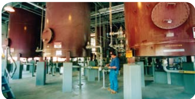
Waste treatment at our DSSI facility
