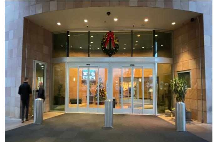
Sensors in entryway (3 sensors, 2 “lanes”)
