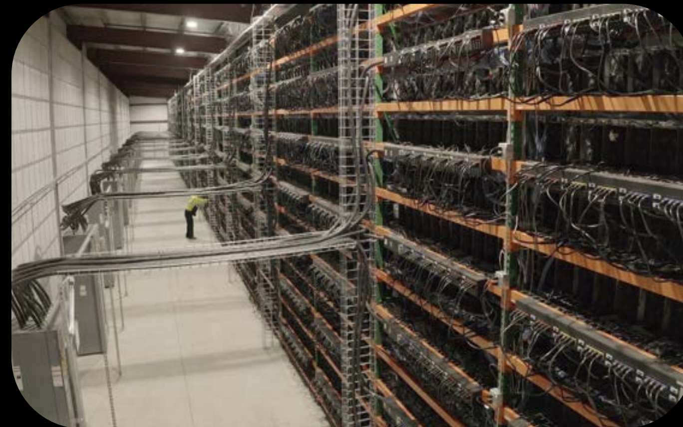
Jamestown, North Dakota Facility 100MWs
