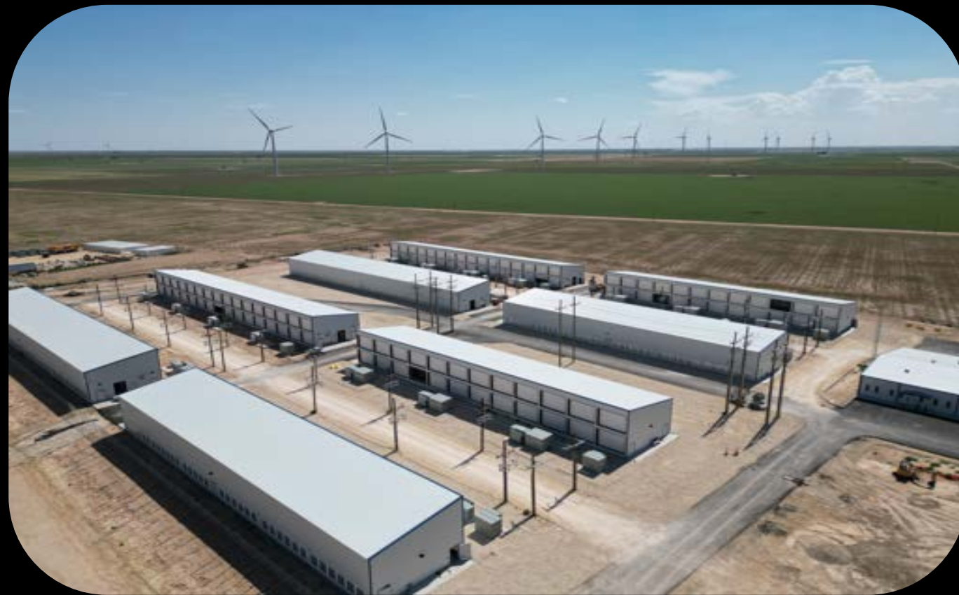
Garden City, Texas Facility 200MWs
