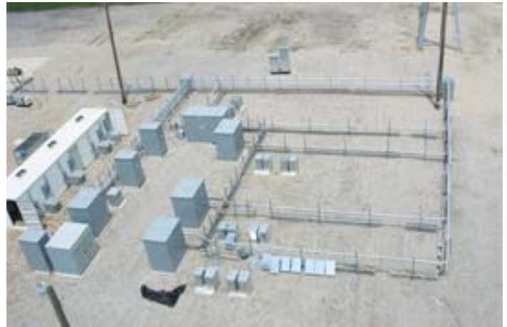
Test layout of the CERTS microgrid at Dolan Laboratory on the campus of
