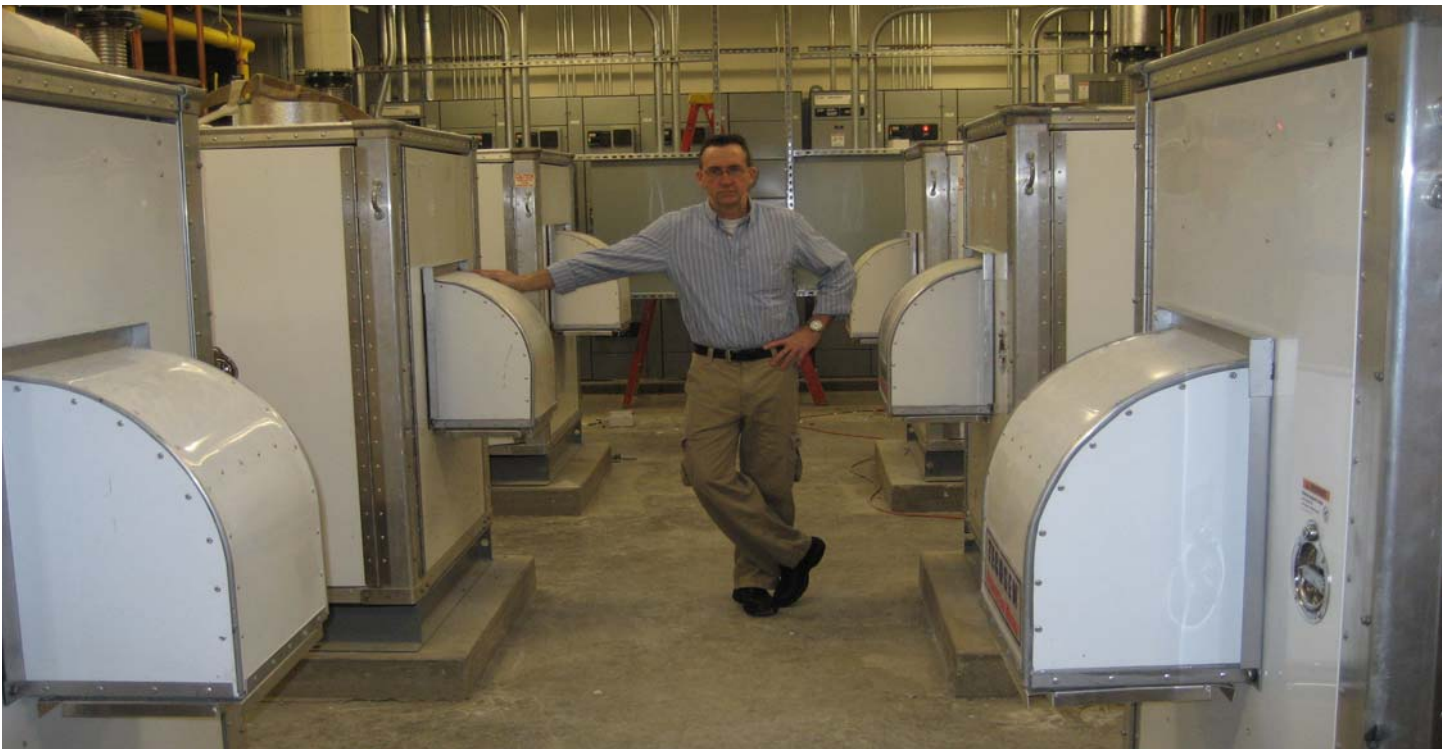
Tecogen President Robert Panora, in a cogeneration plant
