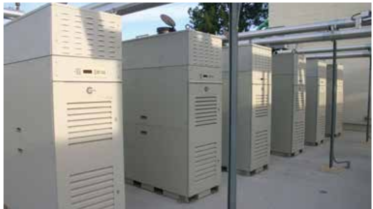
Six Capstone microturbines provide heating and onsite power at this Southern California college.
