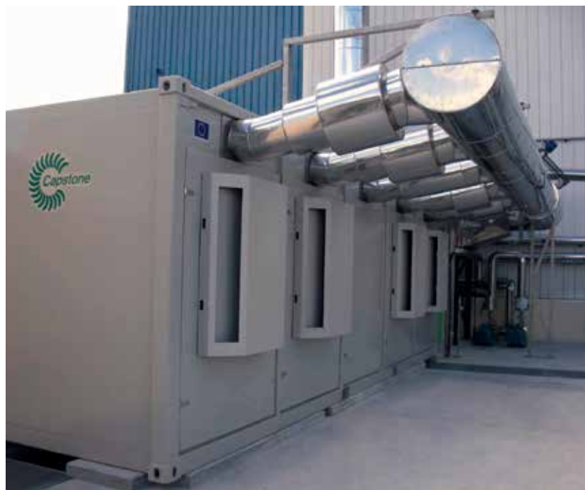
A C800 Power Package is fueled by methane from the treatment of sludge waste (from grape skins and stems) following the distillation of wine to make Cognac.
