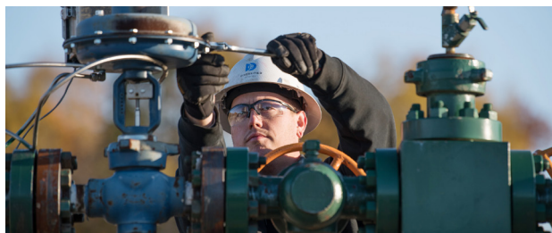
Daily well tending and Smarter Asset Management activities routinely include the use of AVO inspections at our facilities.
