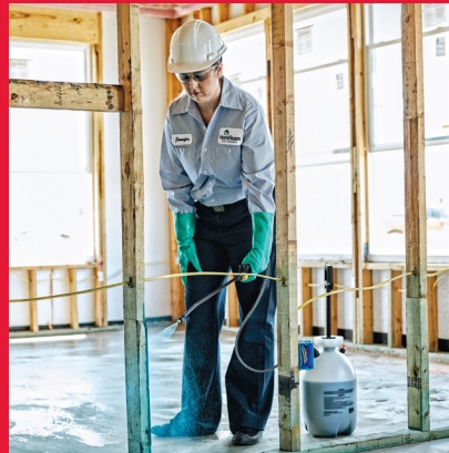
HomeTeam Pest Defense technician installs the TAEXX® tubes in the wall system.
