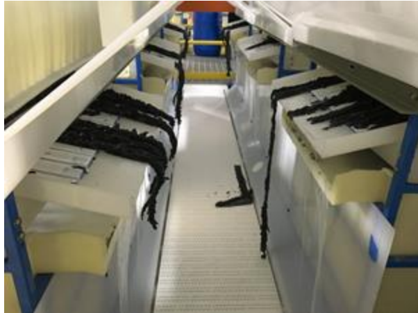
AquaRefining module with six electrolyzer units continuously producing AquaRefined pure lead, flowing like a waterfall of lead infused electrolytes
