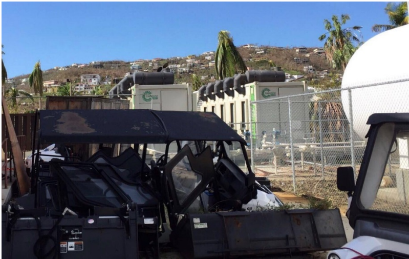
Fully operational Capstone Microturbines on St. Thomas surrounded by debris from Hurricane Irma
