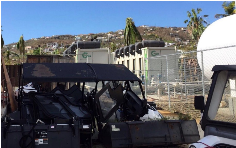
Fully operational Capstone Microturbines on St. Thomas surrounded by debris from Hurricane Irma
