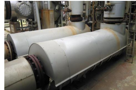
Traditional gas fired heaters
