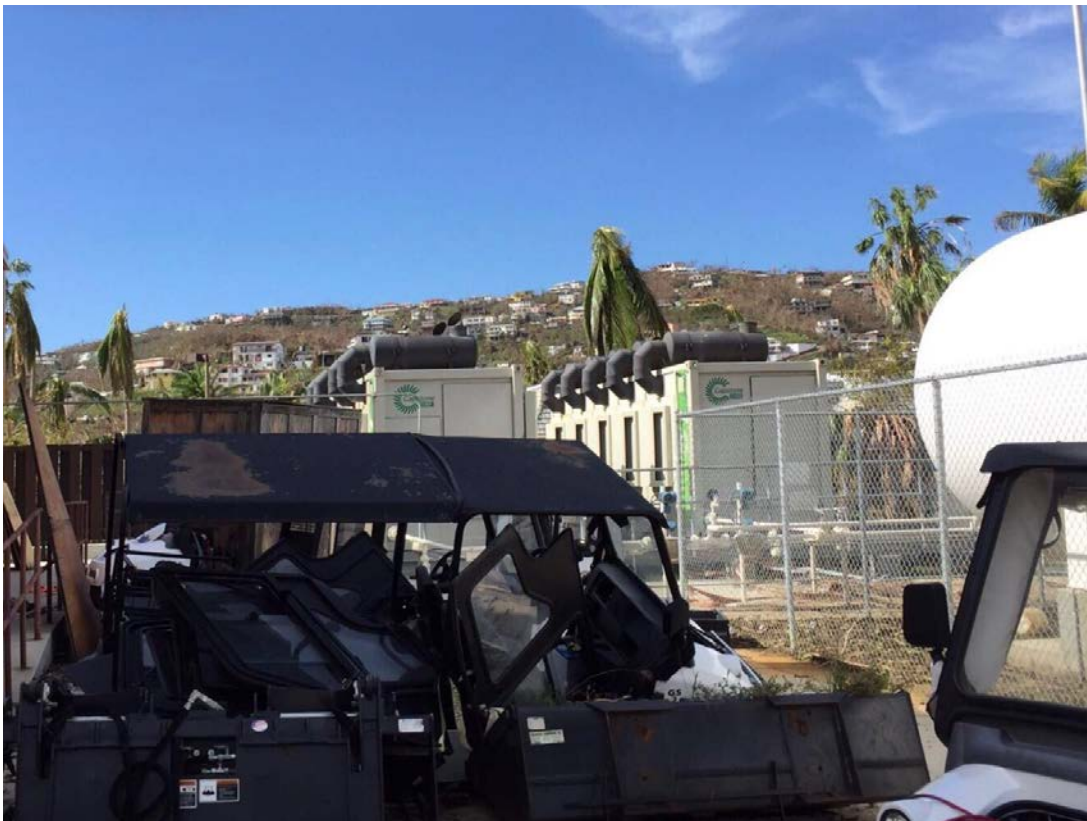
Capstone Microturbines on St. Thomas surrounded by debris from Hurricane Irma
