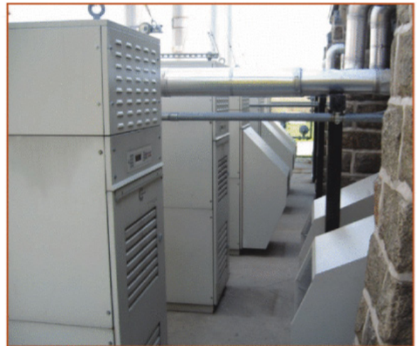
The new system produces 325 kW; is yielding a 47% increase in net heat recovered; and has an overall system efficiency of approximately 83%.
