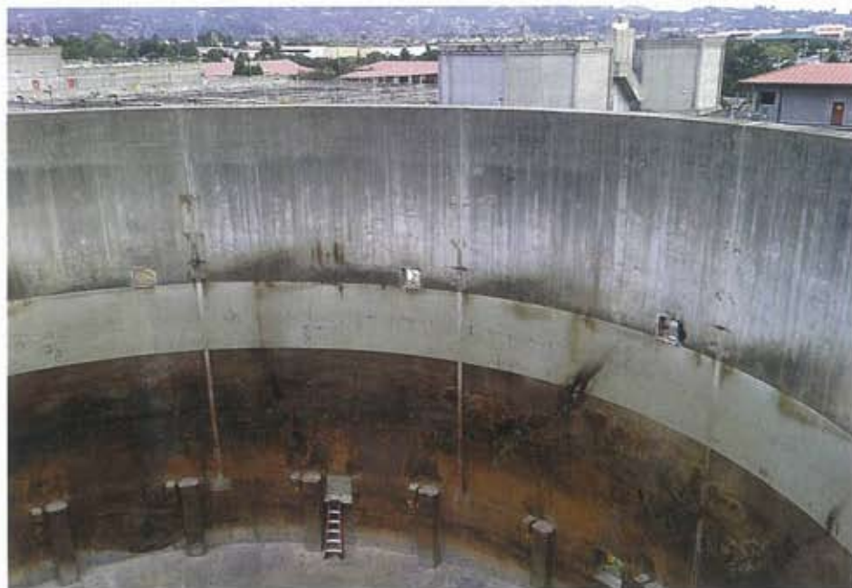
Central Marin Sanitation Agency cleaned out and is upgrading its existing digesters with membrane covers and pump mixing systems (inside of cleaned digester shown above).
